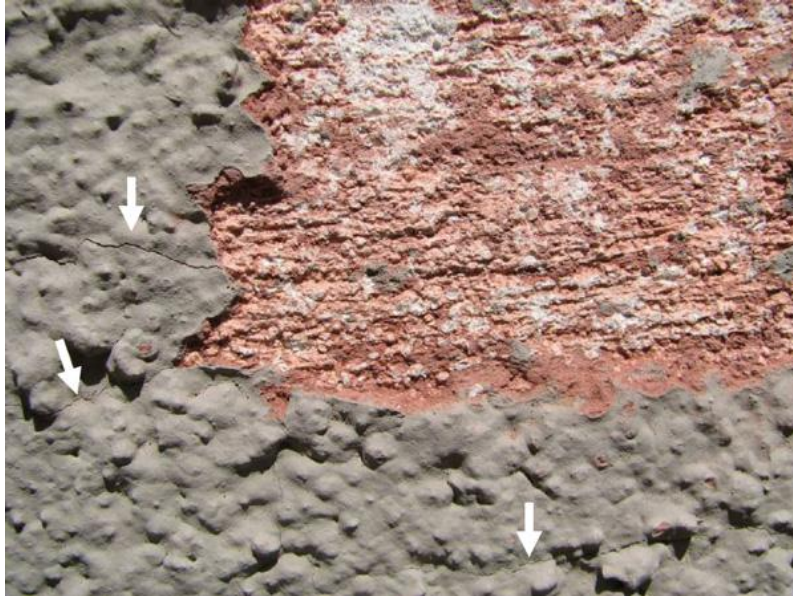
Figure 5 The cracks due to inside VIP expansion (S. Brunner et al, 2012)
